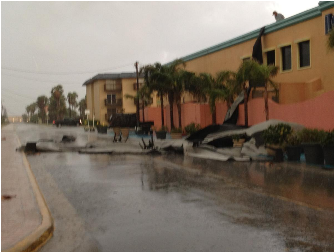
Above: Roofing blown off building associated with Louie's Backyard Restaurant north of the Causeway on the bayside, South Padre Island. Photo credit: Gene Gore, South Padre Island Surfing Company.
