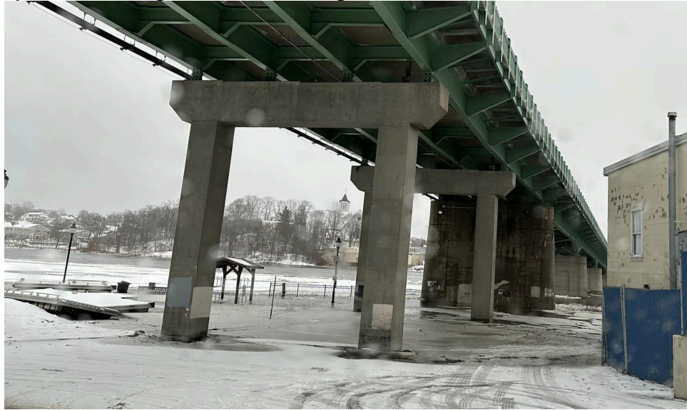
January 13th Flooding in the Kenduskeag Plaza. Picture thanks to Michael Seile Sr.
