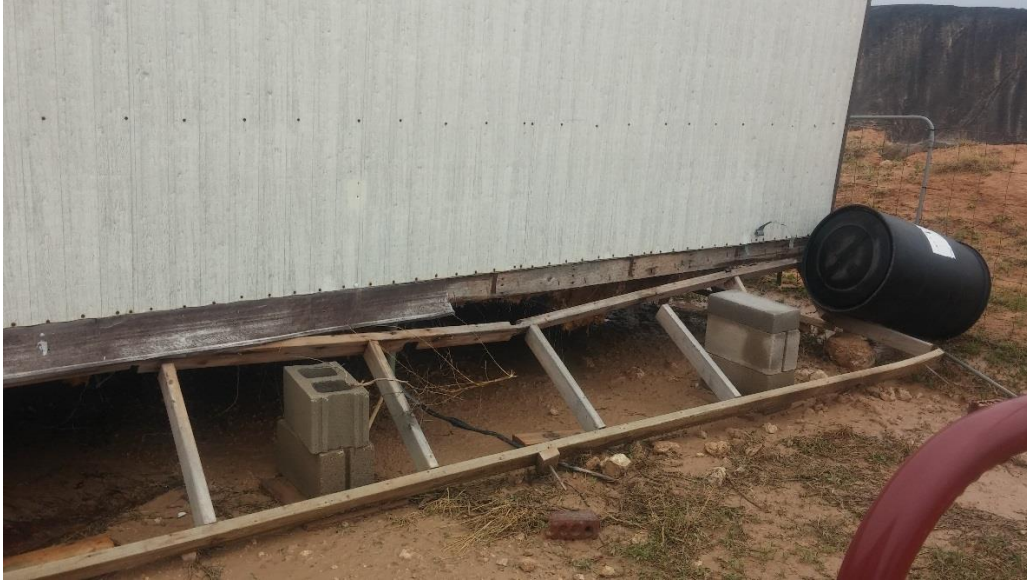
Figure 12 – Mobile home pushed off its foundation (Courtesy of David Hennig).
