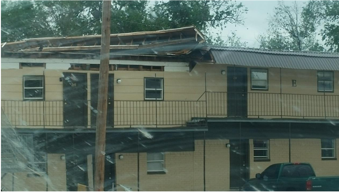
Figure 5 – Damage to Apartment Complex in Big Spring, Texas (Courtesy of David Hennig).
