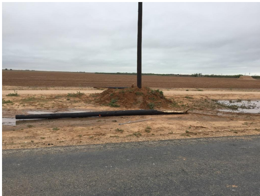
Figure 11 – Snapped telephone pole (Courtesy of Mark Strobin).
