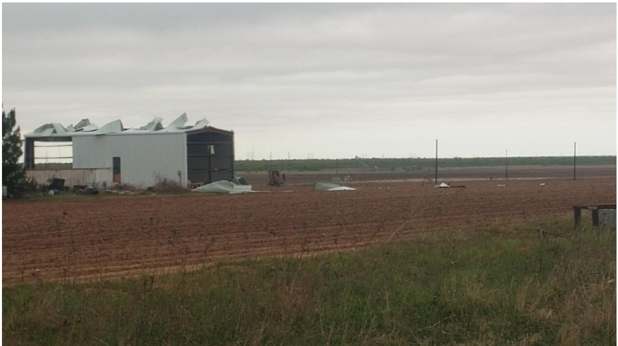
Figure 15 – Barn with its roof uplifted (Courtesy of David Hennig).
