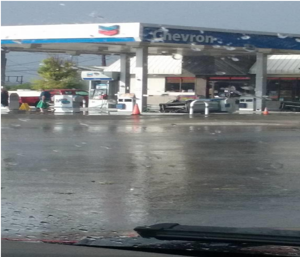
Figure 6 – Damage to Chevron Station in Big Spring, Texas (Courtesy of Laura Murphy).
